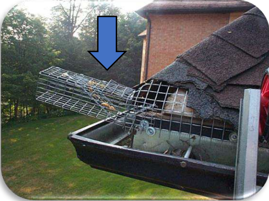
A one-way door (arrow) and exclusionary mesh installed on a squirrel entrance hole on a corner of a roof
