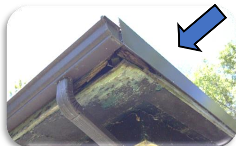
Water damaged wood caused by clogged gutters. Such damage creates openings for wildlife into your home
